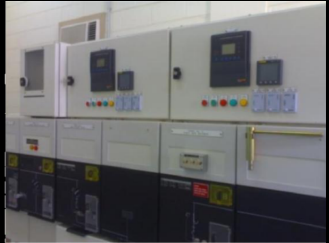
MV switchgear - 4 Standby Generators
