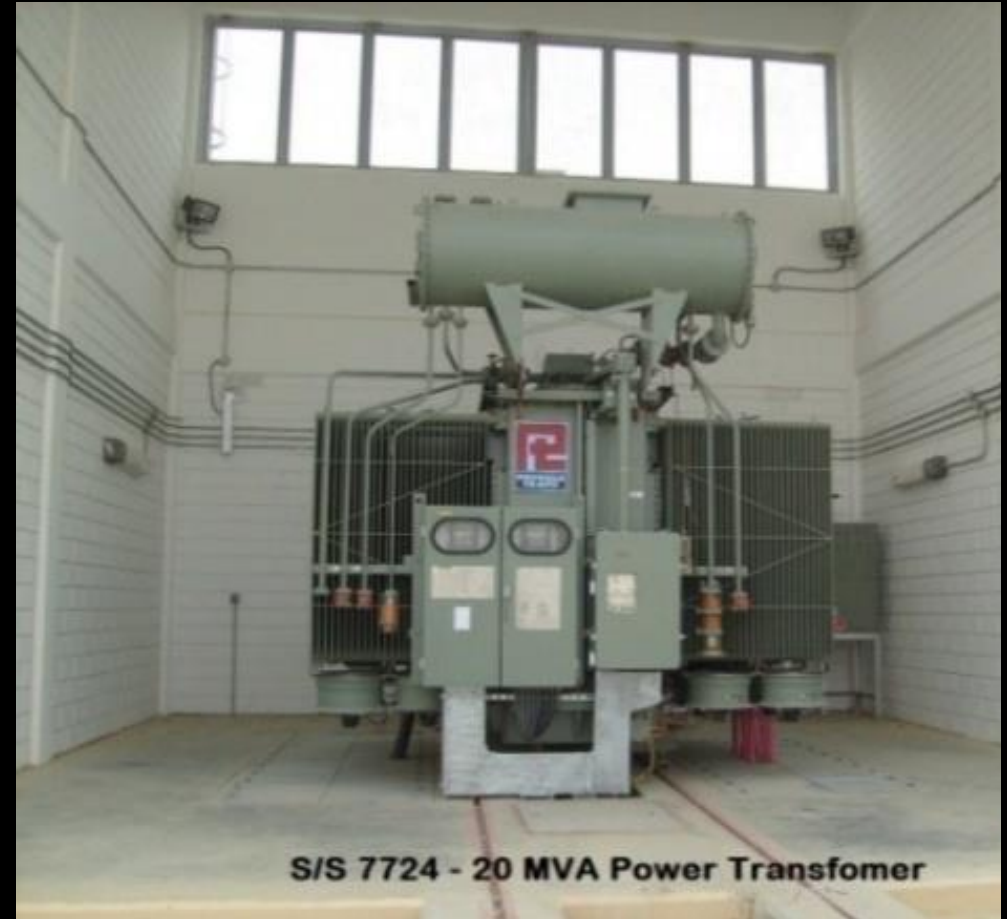
Power Transformer at Al Kharj 7724
