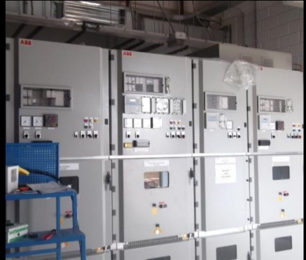
Adam 110 KV substation testing
